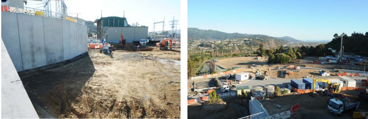
Figure 8: New Platform and Retaining Wall for Pole 3 (left) and New Platform for Switchyard C (right) at Haywards
